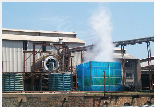
Figure 7: Mist formation in cooling tower outlet air
