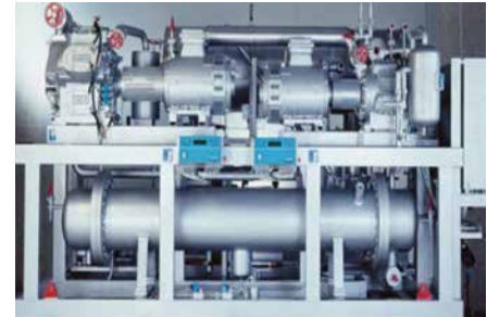
Figure 14: An ammonia-CO 2 cascade system
