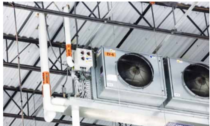
Figure 13: DX ammonia evaporator
