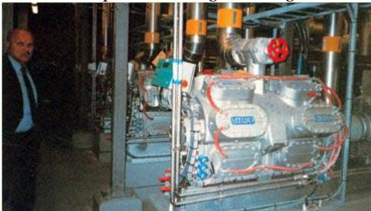
HVAC Plant Room at Oslo Airpopt, Norway
