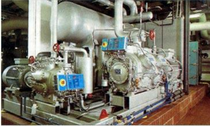
The complete Ammonia Chiller package including electric starter panel and all wiring at the P&T building, Copenhagen.
