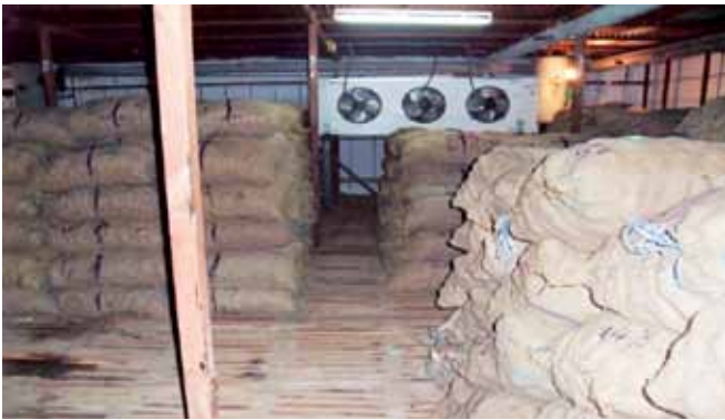
Figure 1: Air coolers (fan coil evaporators)
