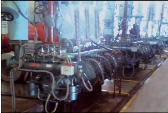
Figure 4 : Bank of four KC93 Kirloskar two-stage compressors.
