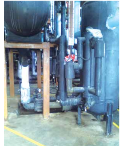
Figure 12 : Ammonia pumps in operation
