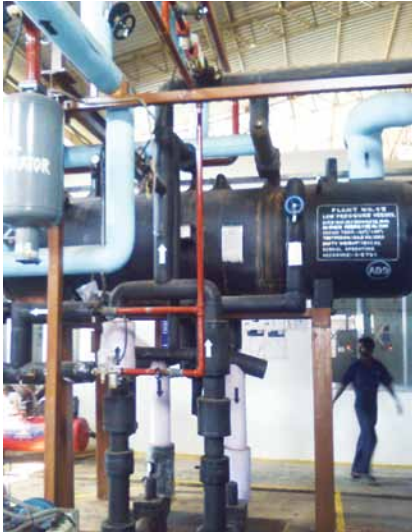
Figure 8 : Low pressure vessel in operation
