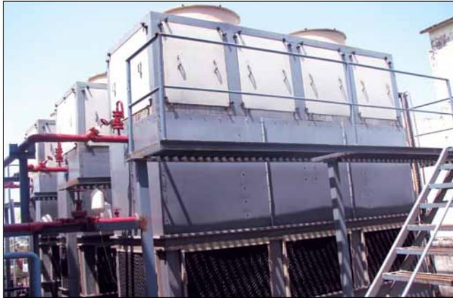
Figure 6 : Evapco make evaporative condensers
